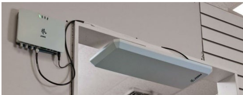
Figure 2-6 Fixed doorway RFID reader
